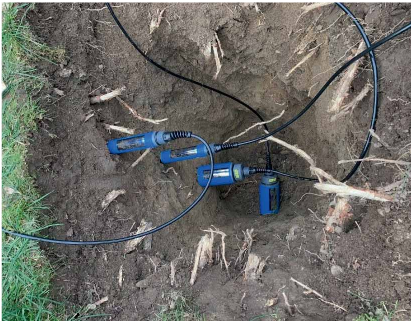
PICO32 (topsoil) and PICO64 (subsoil) in the Reutgraben demo field in Ettlingen
